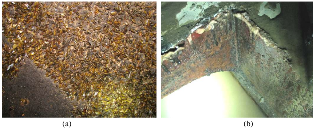
Figure 11 Attachment of golden mussels in 2011: (a) The wall of gate well in the tunnels of ERWSP; (b) The wall of gate well in the scale model tunnels.
