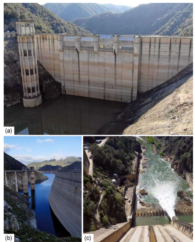
Figure 3 | Outtake structures in Sau reservoir (a) and Susqueda (b) in Catalonia, Spain, on 6 March 2024 and 19 April 2024, respectively. All outtakes in Sau are above the lake level, and the only discharge structure available is the bottom outlet. Only one of the four outtakes in Susqueda remains submerged. (c) Bottom outlet discharging from Sau reservoir to Susqueda reservoir on 12 April 2024. Discharges through hollow jet valves in the bottom outlets can be used to re-oxygenate deep water. Source: Juan Carlos García and Jose Javier Rodríguez-Subiza (ATLL).
